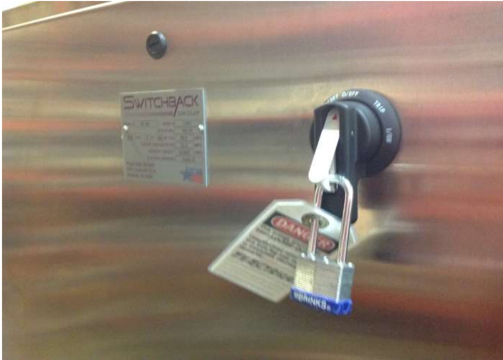
Figure S-1 - Electrical Lockout/Tag Out Point
