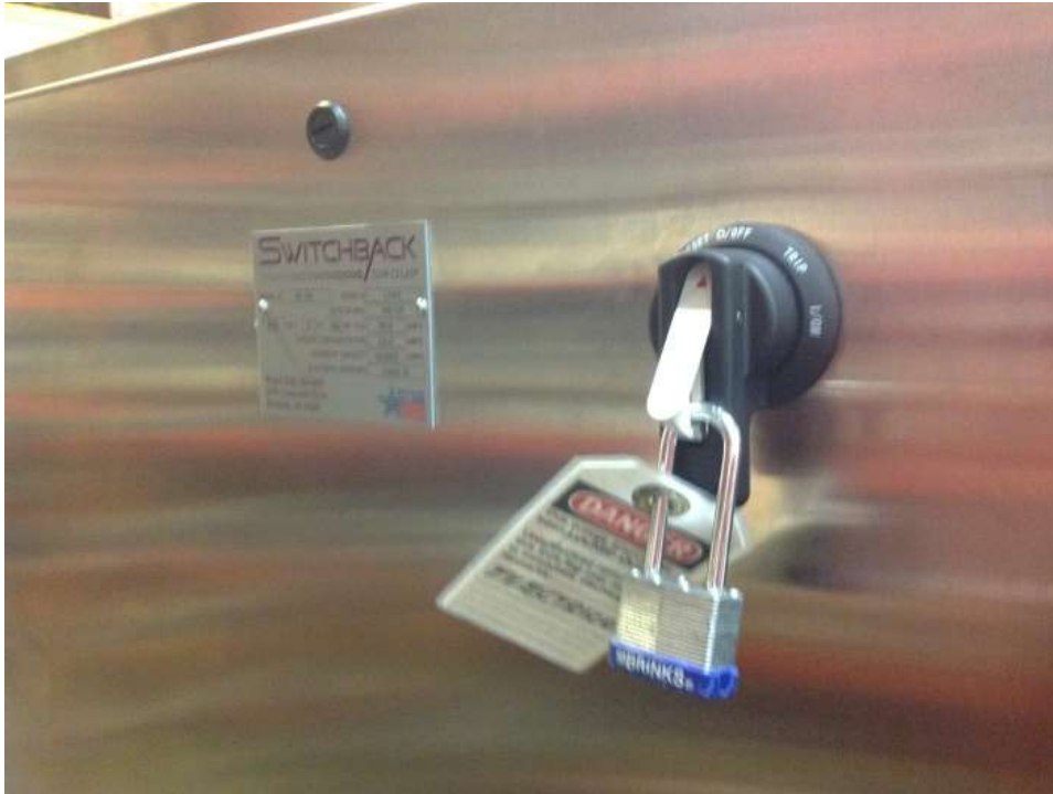
Figure 201 - Electrical Lockout/Tag Out
