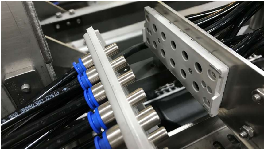
C115 - #5F - Infeed Lane Cartridge Pneumatic Quick Disconnect Removed
