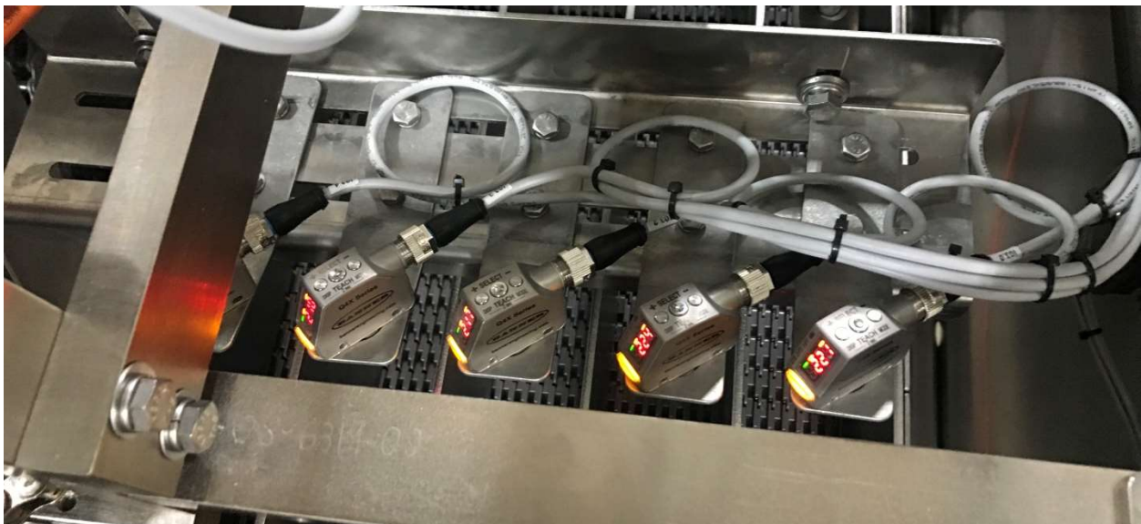
Figure 36 – Infeed Lane Sensors – Top View, Side To Side Adjustment
